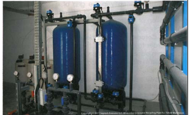
Septech's Grey Water Recycling Plant design is based on four stages of treatment
